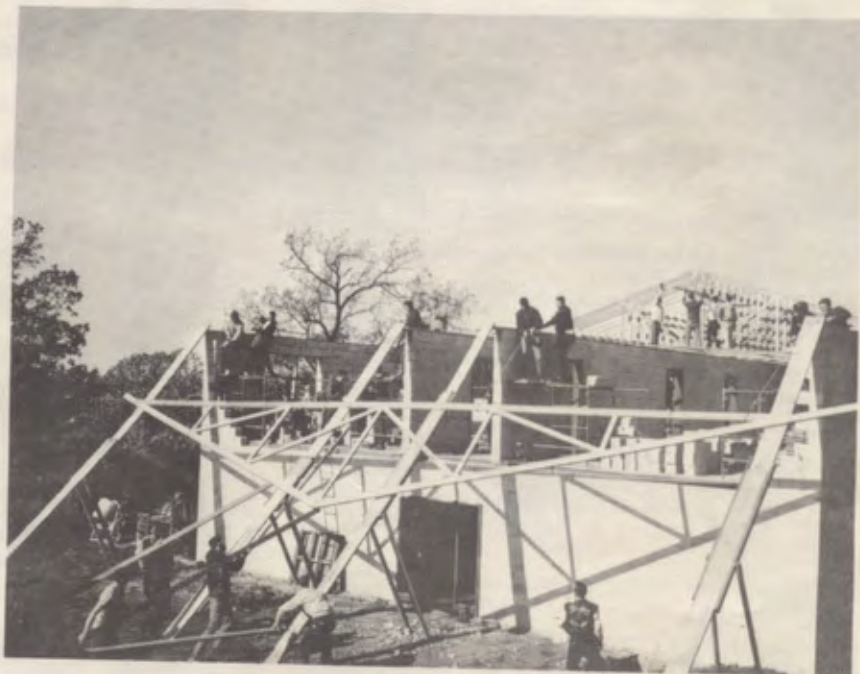
"We're working on the building!" A new boys' dormitory is being built right near the present one. This building will accommodate about fifty boys.
